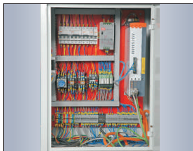
Electric control panel (for NC version)
